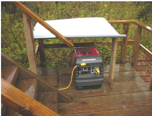
Good generator installation
