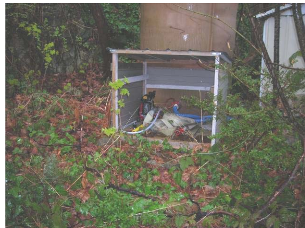
Fire Pump at a residence
